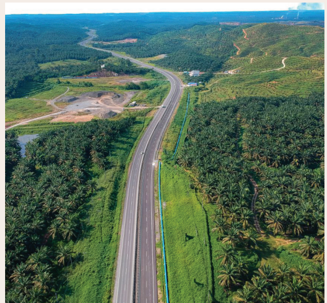
Image 1 Expansion work of Pan Borneo Highway, which will be expected to be completed by 2027.
